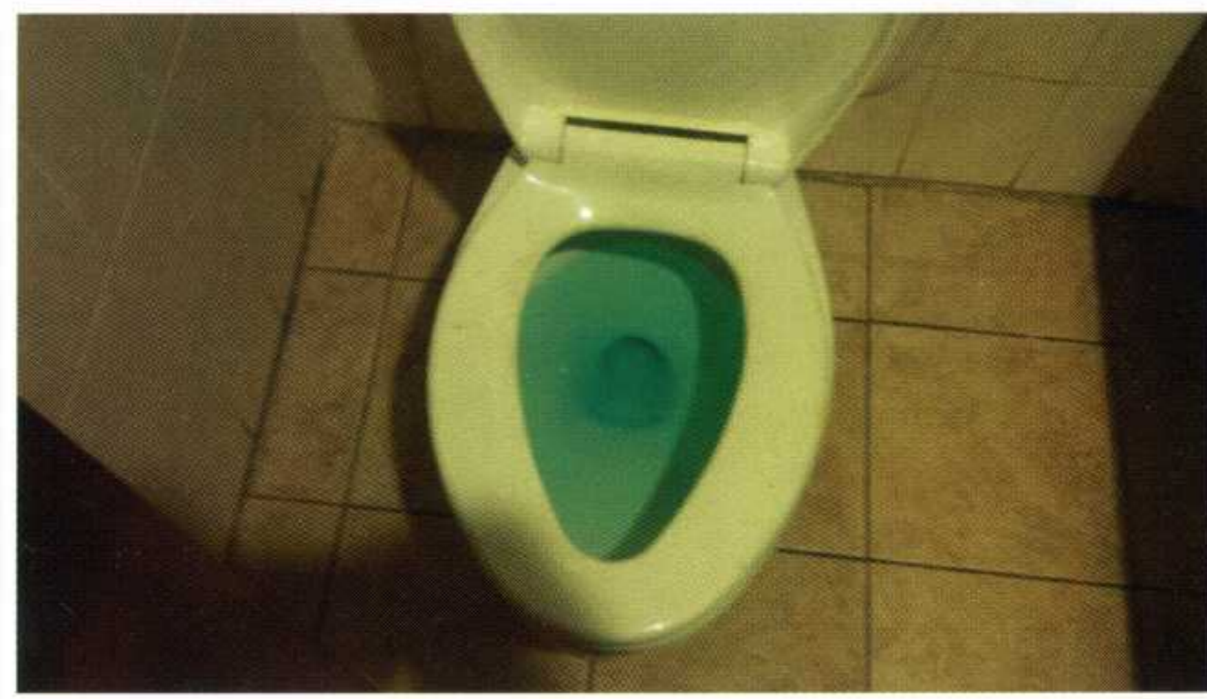
A blue dye is injected to distinguish this non-potable water from potable water.
