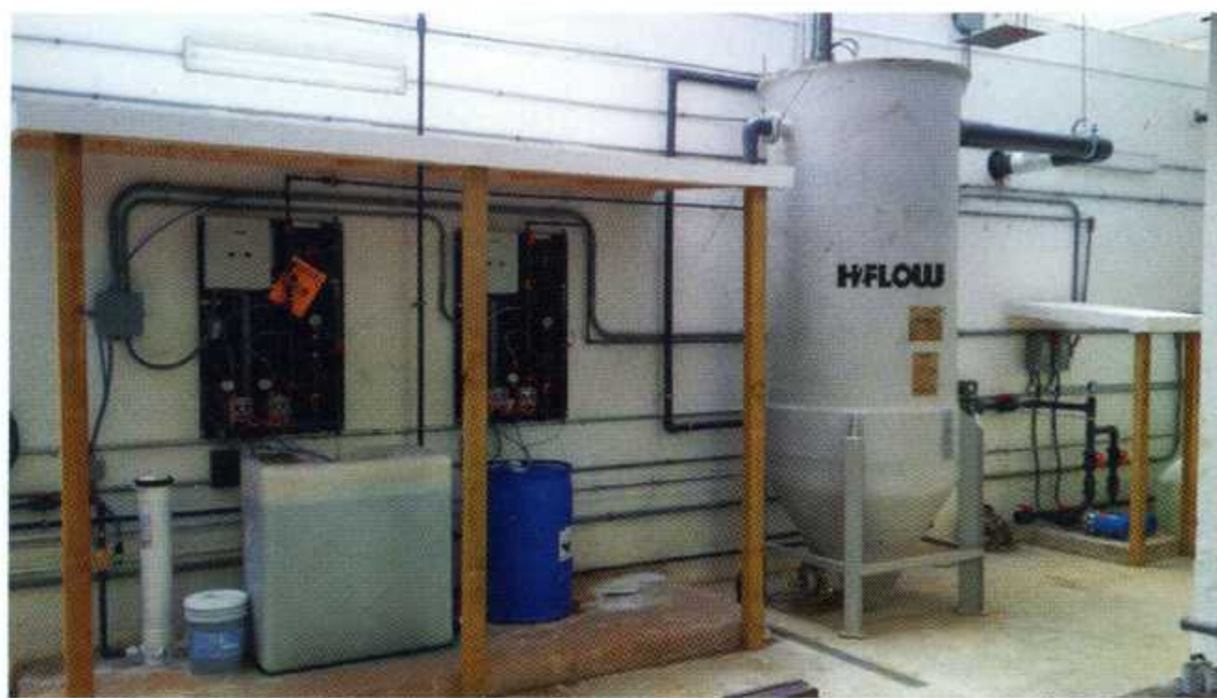
H2Flow provided all equipment and training for the effluent reuse system.
